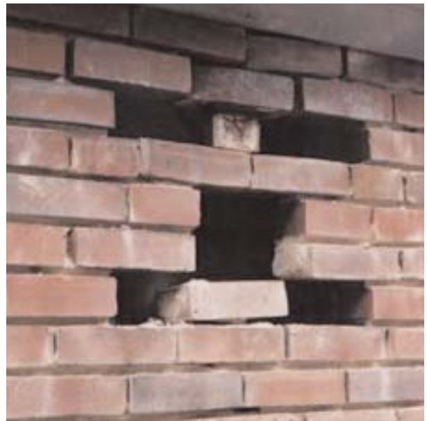
Deteriorated gallery brick screen.
